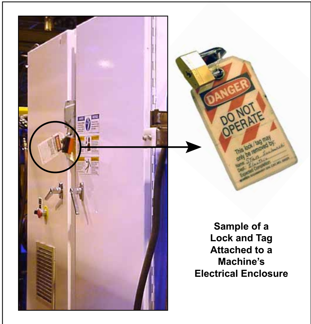
Figure SAFETY-1: Lockout/Tagout on the Main Electrical Enclosure
