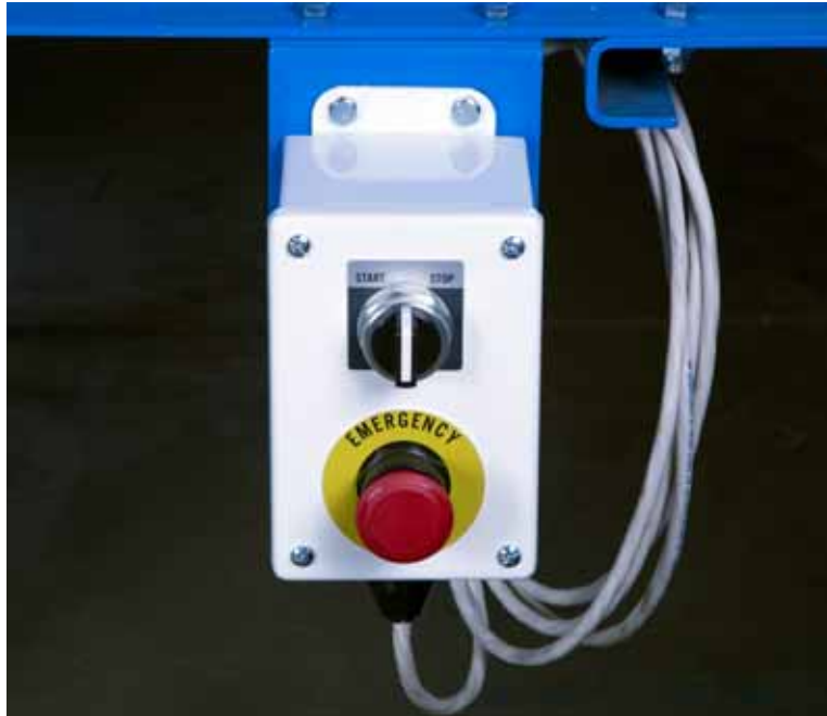
Figure 4-19: Control Station on Powered Skewed Conveyor
