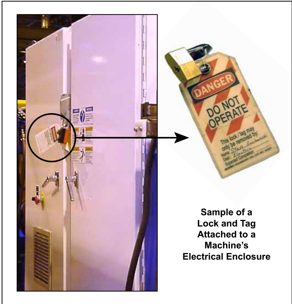
Figure SAFETY-1: Sample of a Lockout/Tagout Mechanism on an Electrical Enclosure
