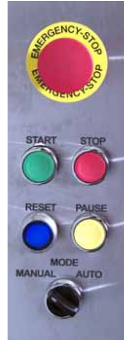
Figure 4-16: Mechanical Controls on Operator Interface Panel
